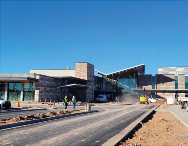
Pictured: Front entry construction of the Dilkon Alternative Rural Health Center in Dilkon, AZ. The center, serving the Navajo Nation, consists of over 30 departments and 600 rooms and offers emergency and diagnostic services. The facility was completed in February 2022.
